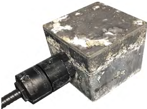
Example of corrosion on Sentinel cable gland
