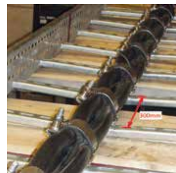
After short circuit test
