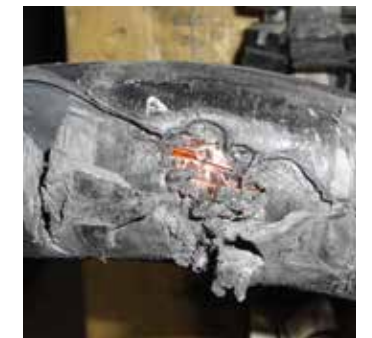
Major cable damage caused by thread contact
